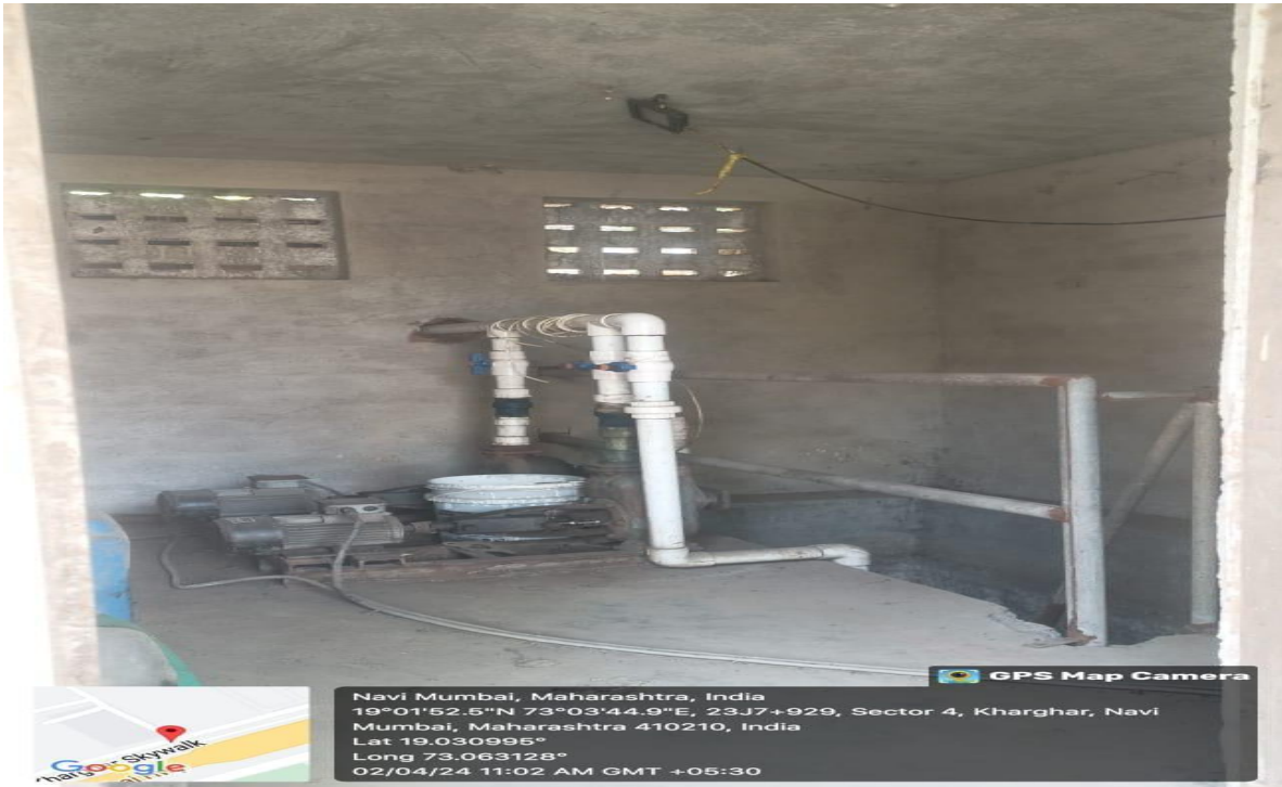
Sewage treatment plant STP (Water recycle)
